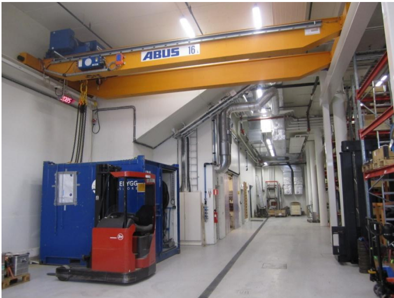
Figure 6 Container and testing area with overhead travelling crane
