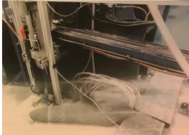
Figure 4.21: Cables near punching machine at Glamox Company
