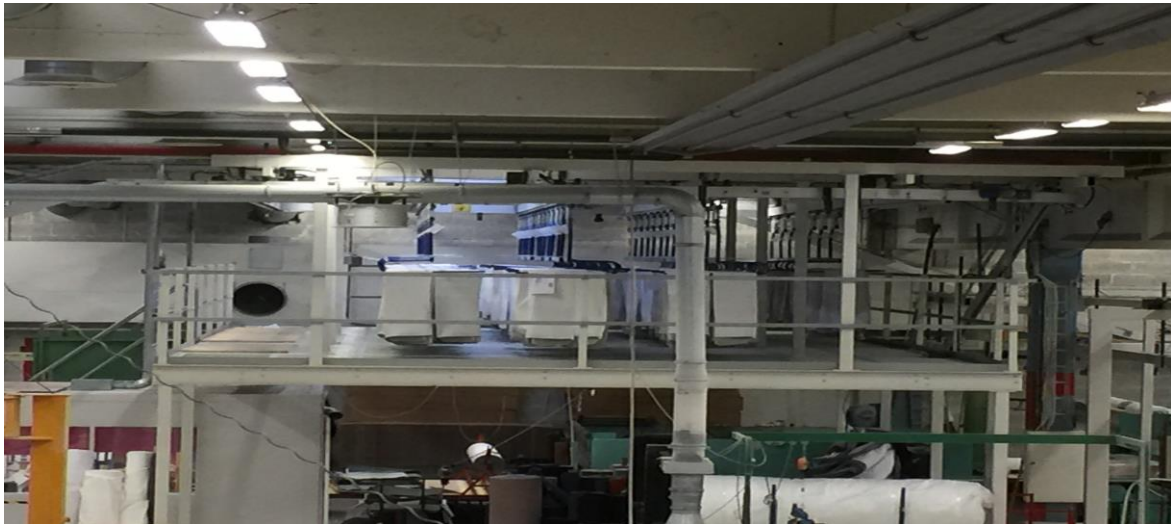
Figure 34. The cover buffer in the cover production area
